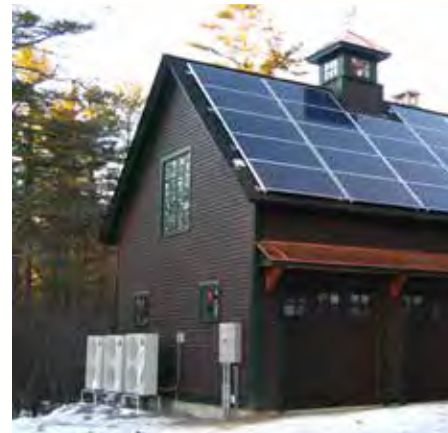
The heating system, installed and designed by ARC Mechanical Contractors, includes three Mitsubishi Electric MXZ all-weather air-source heat pumps.
