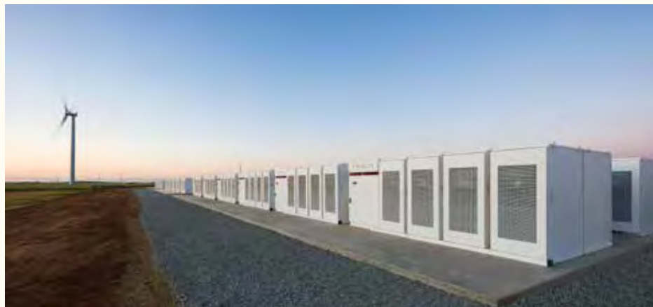
Tesla battery system in Australia. Images via Hornsdale Power Reserve and Tesla on YouTube.
